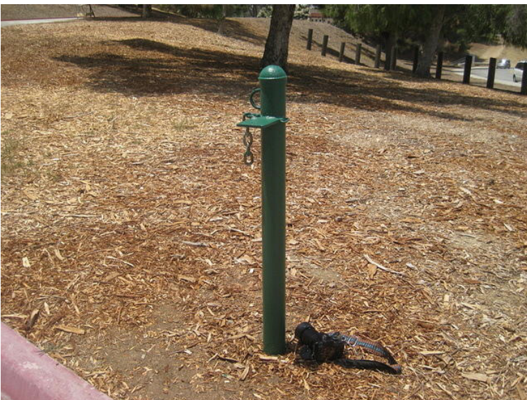
One of the poles by the swinging gate that also needed re-painting.
